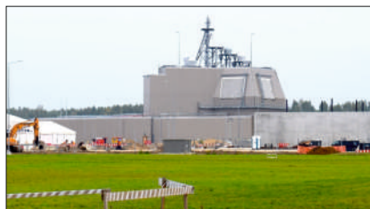
Polonya Aegis Ashore Füze Savunma Tesisi Poland Aegis Ashore Missile Defense Facility
